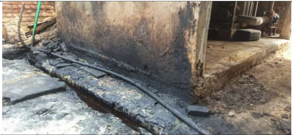
Poor housekeeping near ETP Area
