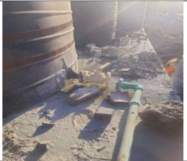
Leakage in bottom valve of effluent storage tank
