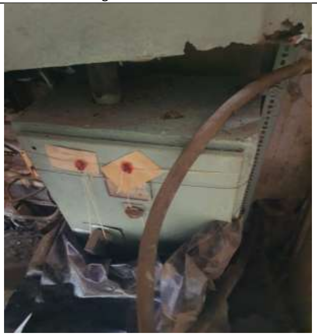
Sealed electric box
