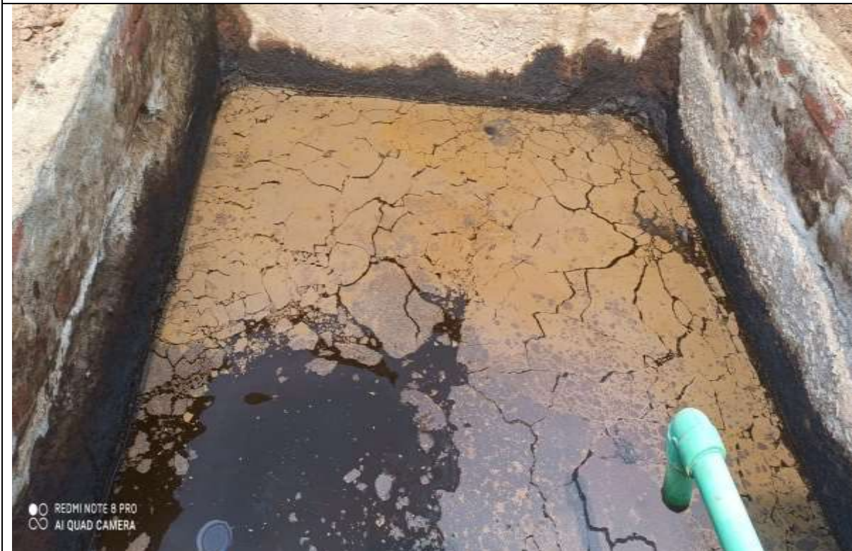
settling tank of ETP
