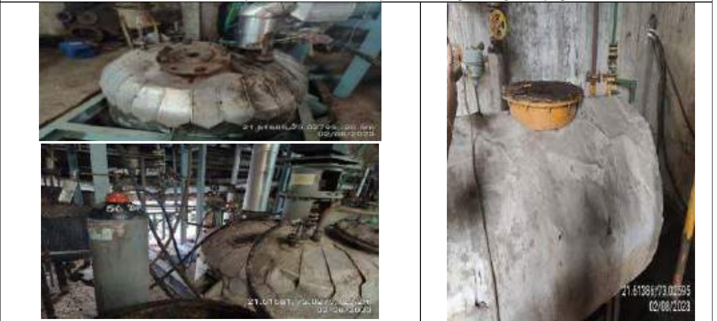
0.7 kl SS reactor, 6 KL reactor connected with nitrogen cylinder and electric hot oil unit
