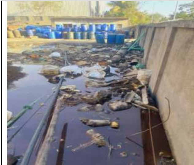
w/w ponding near boundary wall within premises
