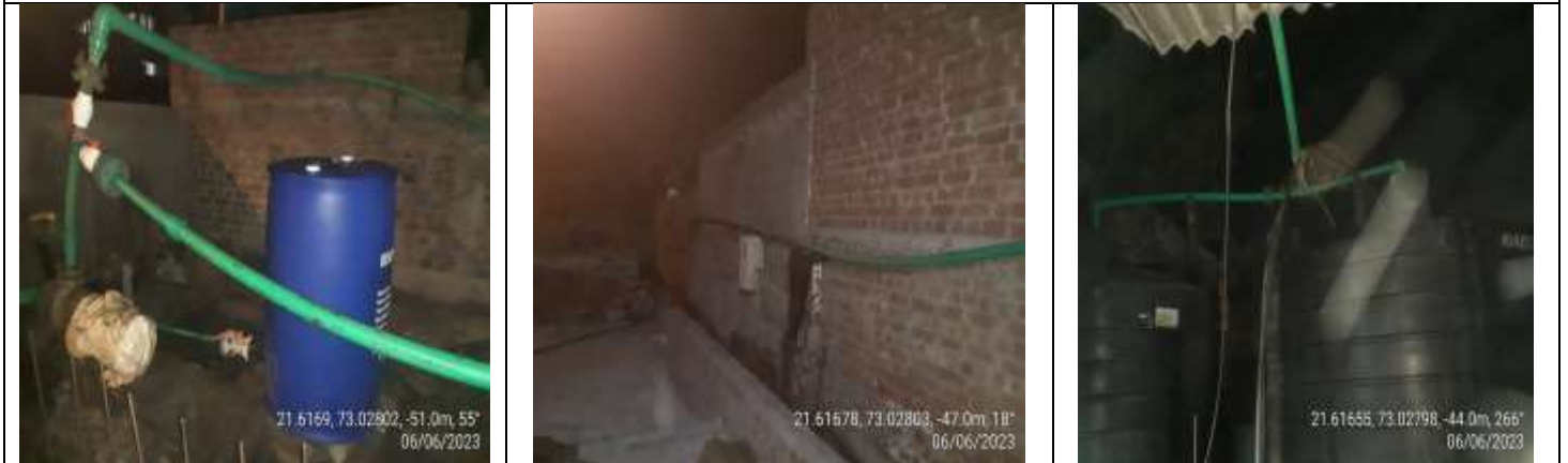
Generated w/w from the manufacturing process is been simply passing through ETP and the same is been transfer to final treated w/w holding tanks through provided fixed pipe line system.
