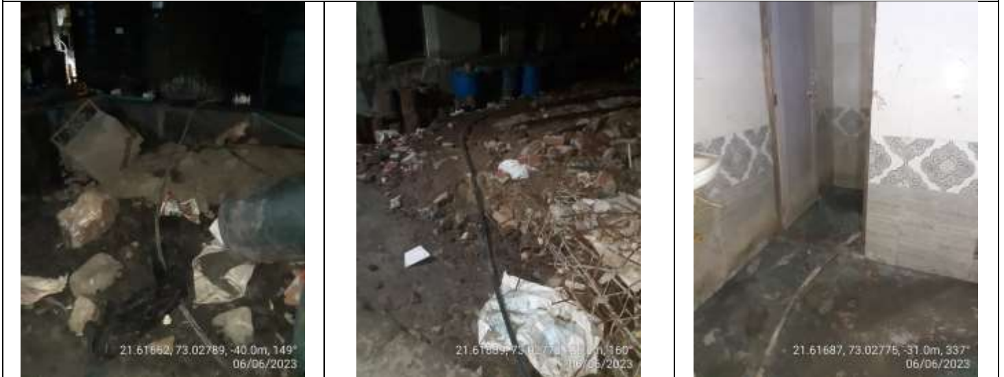
Unit has provided outlet pie line with valve system at the bottom of third holding tank which is connected with @ 50 to 60 meter length of flexible pipe line up to the bathroom.
