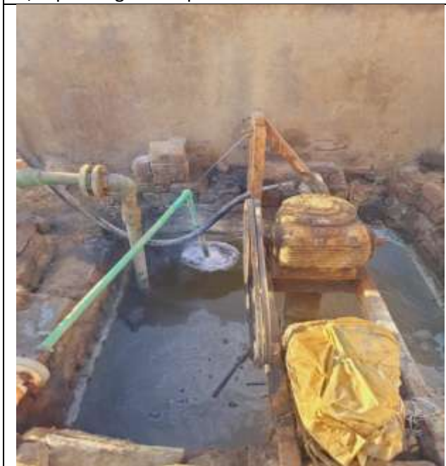
Neutralization tank of ETP
